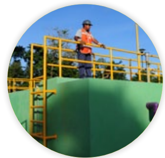
Cancun Airport's waste water treatment plant
